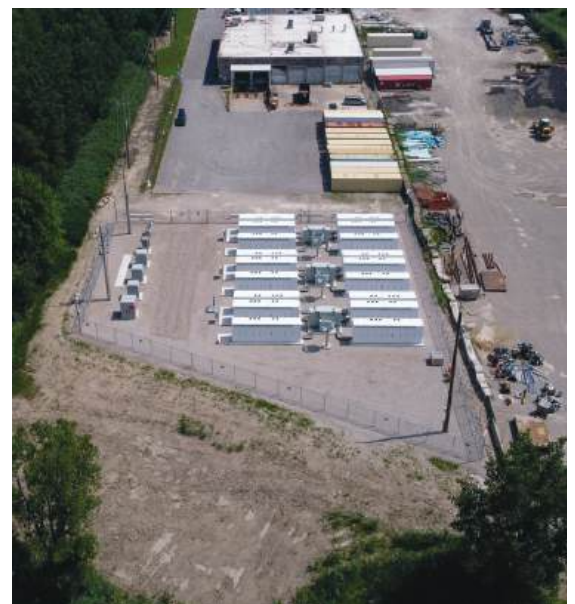
CGD's Walker BESS 4, 5, and 6 Project
